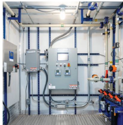
Main control panel
